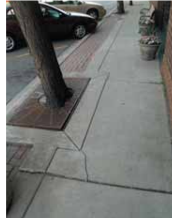
Deteriorated paving on Center Street
