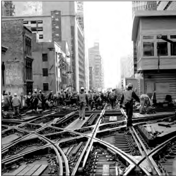
Crews worked around the clock over the course of four weekends to replace deteriorated rail ties and track components at one of the busiest rail junctions in the U.S. – CTA's Tower 18 –located at Lake/Wells. Five of CTA's eight rail lines travel through this junction each weekday.
