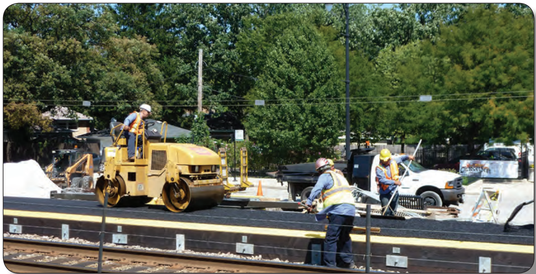
Workers resurface the platform at the Edgebrook Station on the Milwaukee North Line.
