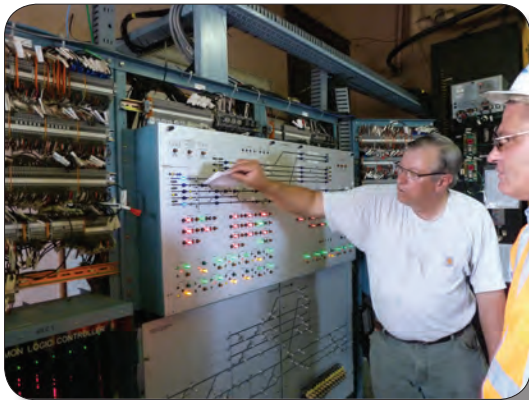
A Metra signal maintainer explains the function of a local control panel at Kensington.
