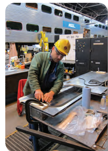
A new seal is placed around a window as part of the Amerail railcar rehab at the 49th St. Shops.
