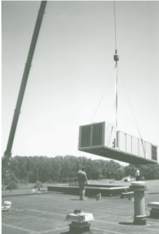
Pace recently completed a new HVAC-Project at its South Division Facility in Markham
