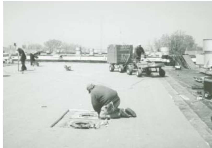
Pace completed a $1.2 million dollar roof project at its West Division garage in Melrose Park.
