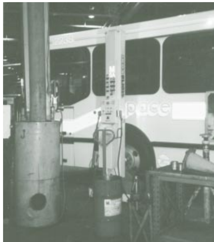
Pace recently completed a bus lift replacement project at its West Division Garage in Melrose Park
