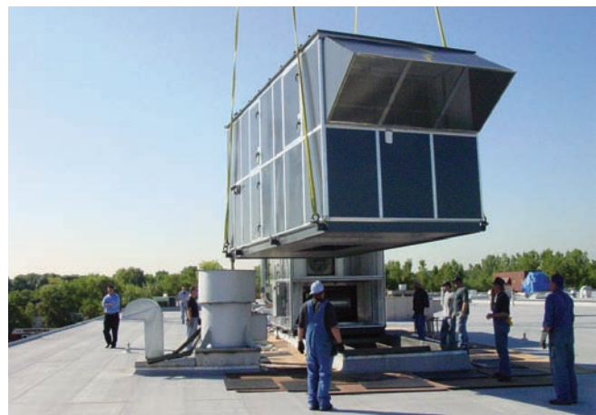
Pace’s South Division is 20 years old and was in need of a major HVAC replacement. This system replacement was completed in 2005 for more than $700,000.
