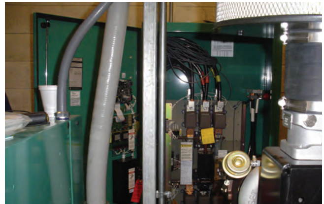
Pace installed an emergency generator at its McHenry County Paratransit Garage. This equipment helps avoid service disruptions due to power outages.
