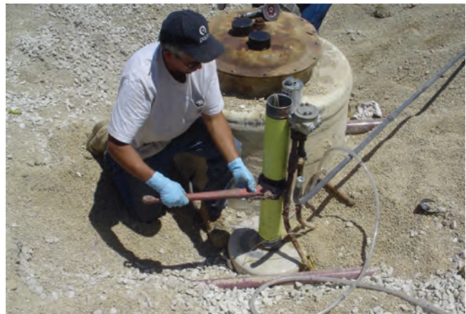
In 2007, Pace completed repairs to its underground storage tank in Bridgeview in Spring, 2007.
