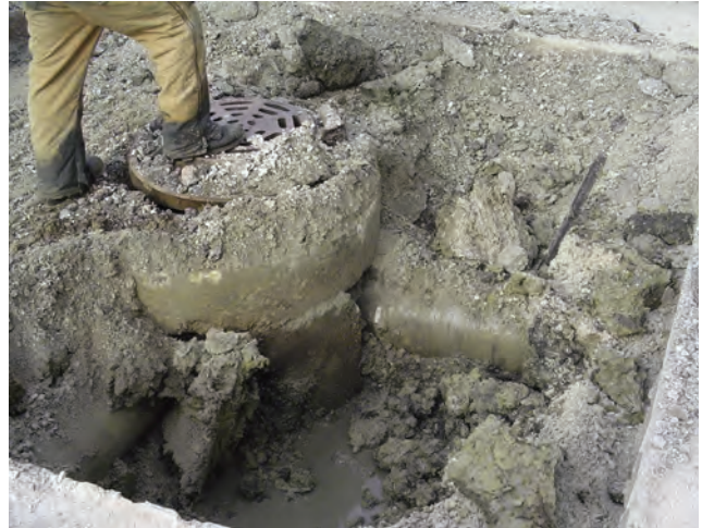
This catch basin collapse is a result of deferred capital investment.
