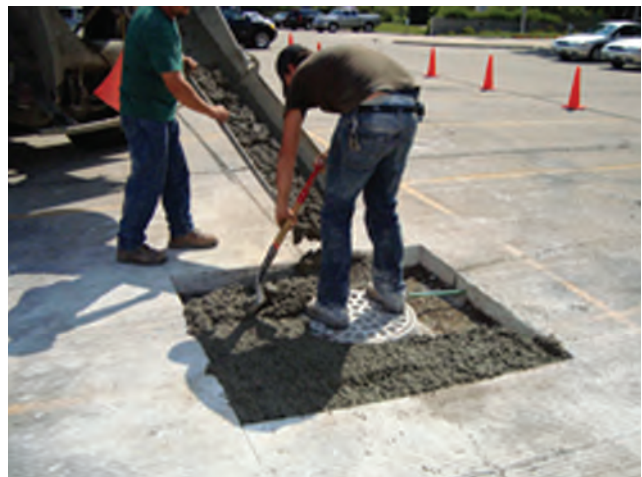
Pace replaced a storm catch basin at North Shore Division in Evanston.
