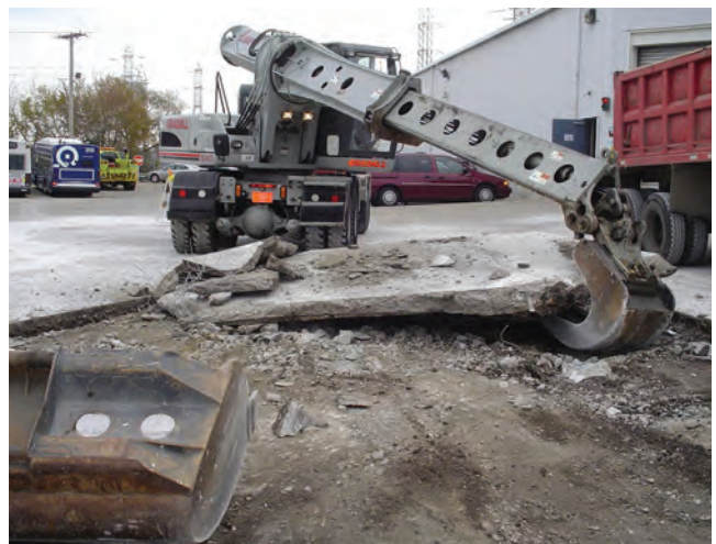
Pace replaced the concrete at its Northwest Division in Des Plaines. This pavement was very deteriorated and doing damage to our buses.
