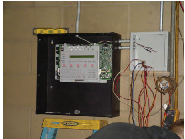
Pace replaced the fire alarm panel at Heritage Division in 2008. This project is part of a $1.0 million replacement program awaiting new capital funding.
