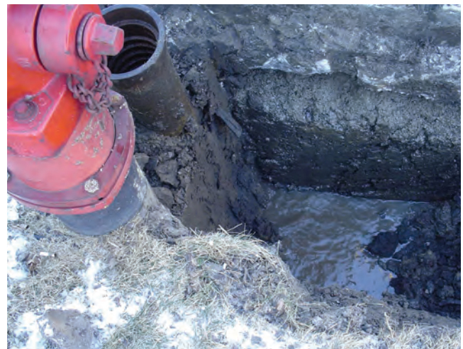
A new fire hydrant was installed at South Division in Markham after the hydrant failed.
