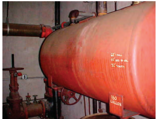
The fire pump tank at South Division is in need of replacement. This will be done once new capital funding is secured.
