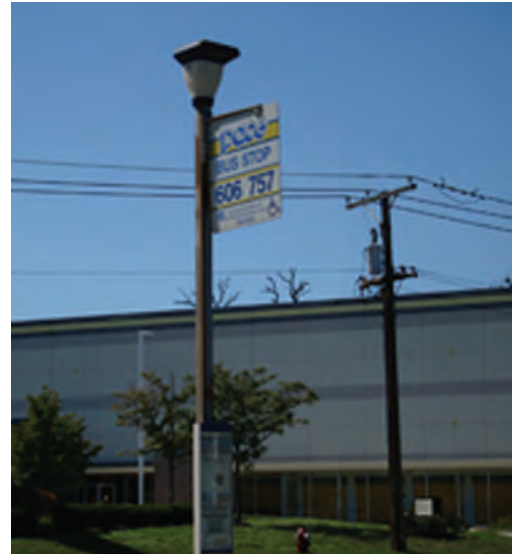
This solar powered bus stop sign provides light to passengers waiting at bus stops.
