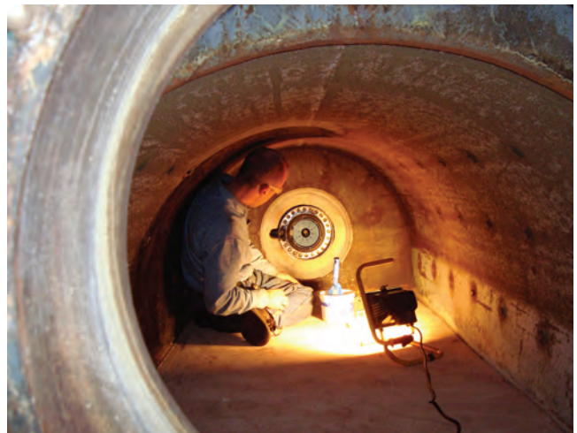
A new Burnham boiler blast tube was replaced at River Division in 2009.
