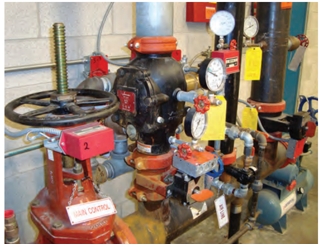
The Dry Valve System was replaced at our McHenry County Garage in 2009.
