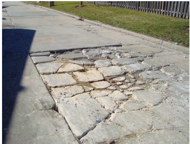
Pace has millions of dollars of concrete and asphalt repairs to make.
