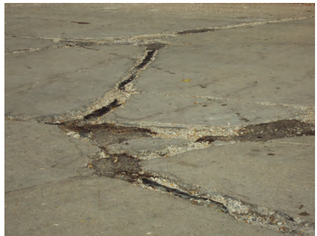
Concrete replacement is a very costly improvement and deferral of capital dollars is causing a great backlog of the work.
