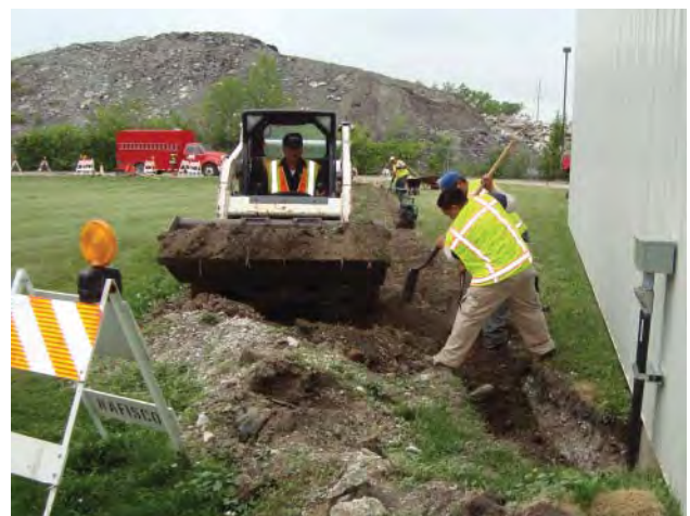
In 2010, Pace repaired six diesel tank sump enclosures at its North Shore garage.
