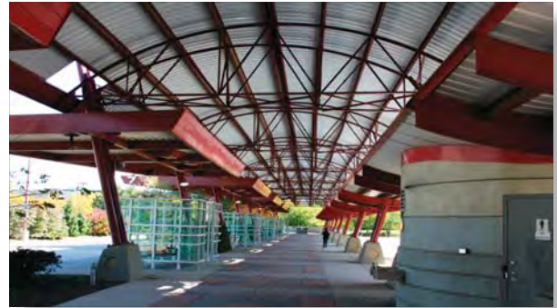
Pace will be performing structural steel rehab to its Northwest Transportation Center in Schaumburg in 2013.
