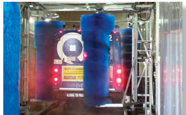
In 2012, Pace replaced the bus wash system at Heritage Division. Portions of this building are nearly 90 years old and dates back to 1926.
