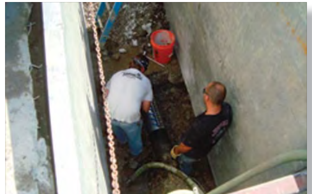
Predictable state funding is critical to address State of Good Repair projects- West Division water main break in 2013.
